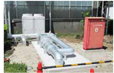
Above-ground water supply pipes
